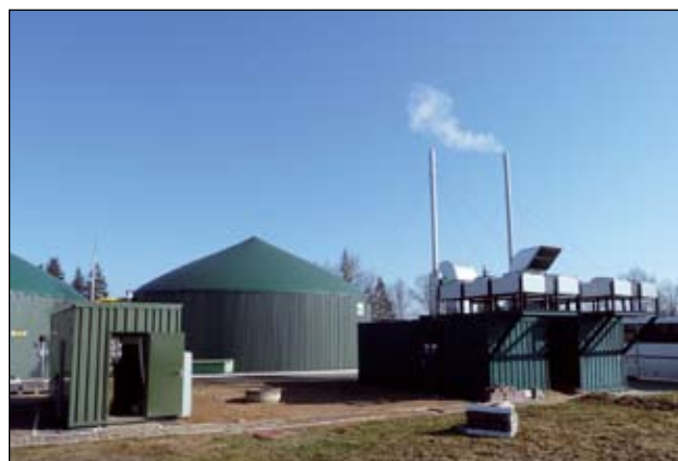
Belarusian biogas plant. Photo: Lars Rydén.
