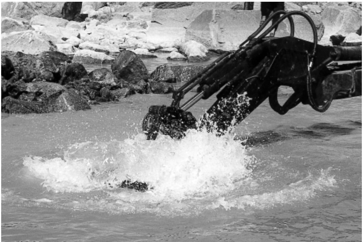
Building and construction work may lead to pollution of water which is considered in environmental impact assessment (photo, Inga-May Lehman Nådin).
