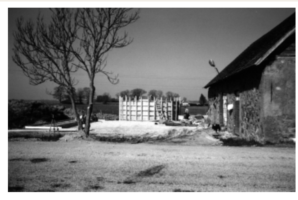
Figure 8.8. The new manure pad at the Māo farm, Estonia (Swedish University of Agricultural Sciences, 1998).
