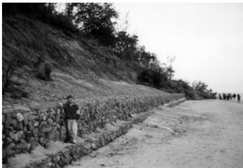
Figure 2.2. Cliff coast protected by Gabion's seawall. Material has fallen from the cliff and reached the sea over the seawall construction. Groundwater impact is intensified by inadequate water management of the developed area located on the cliff which consists of many sand and clay layers. Jastrzebia Gora, Poland.
