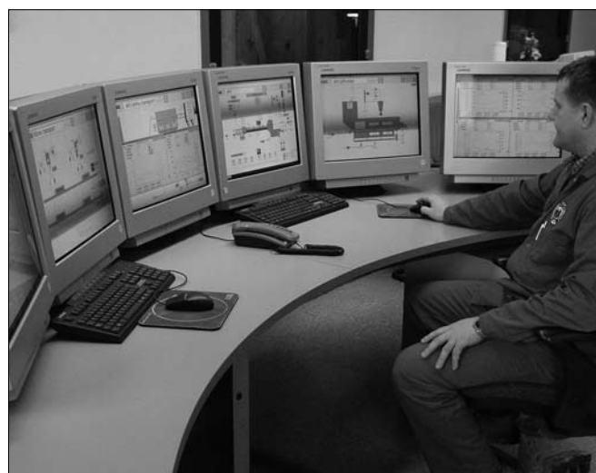
Figure 1.4 The control room.
