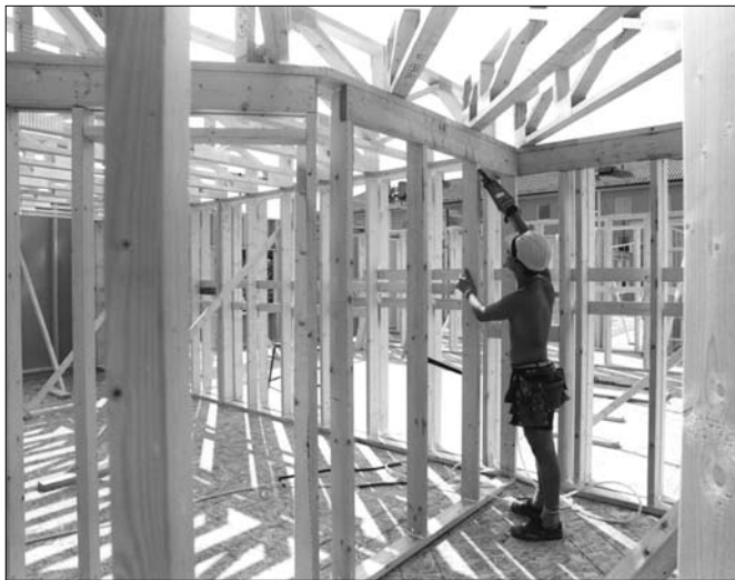
Figure 3.2 Environmental management in the building sector has resulted in some remarkable results. One of the many advantages of multi-storey wooden houses, here being built outside the Swedish city of Norrköping, is many times lower consumption of the natural resources, less handling of heavy material, easy transport etc. Photo: Holger Staffansson, Skanska.
