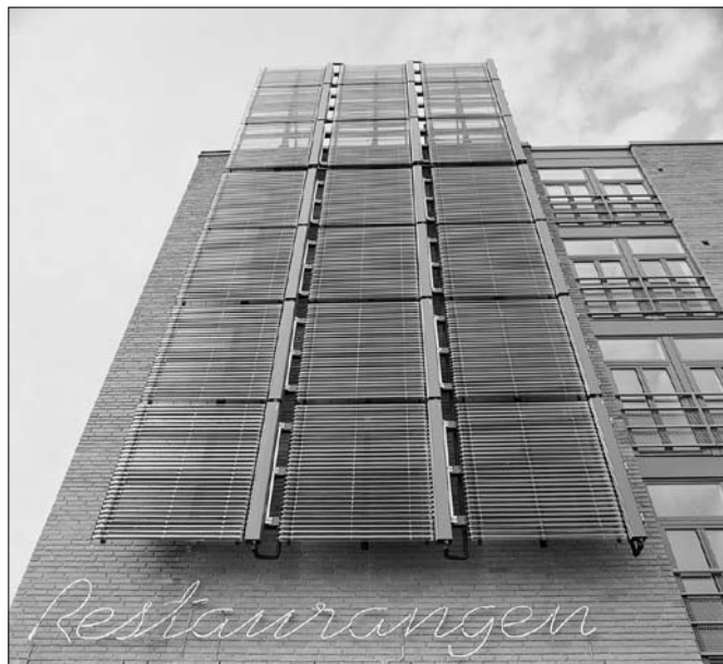
Figure 4.3 A solar collector balcony (Example 3). This balustrade is used both as a solar panel and as a balcony balustrade. The Vitosol 200 model is found in the City of tomorrow (Bo01 exhibit in 2001) in Malmö. Photo: Viessmann Werke GmbH & Co KG.
