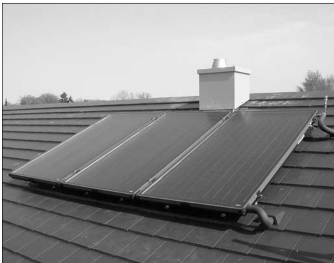
Figure 3.4 Solar panels. Warm water may be provided by using solar panels, a solution which is growing more economically competitive as the technology develops.
