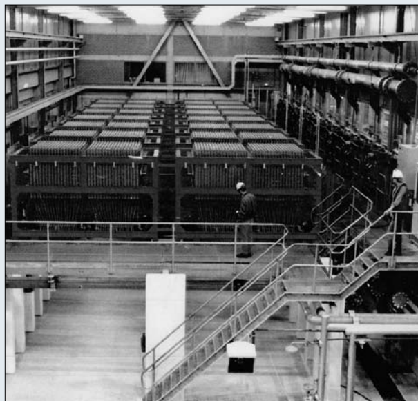
Figure 7.1 Chlor alkali industry. View of a membrane cell room equipped with bipolar electrolysers [source: the BREF document].
