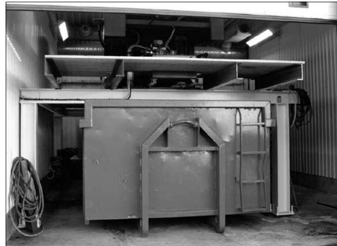
Figure 1.2 Chamber filter press for dehydration of fat from the fat separator.
