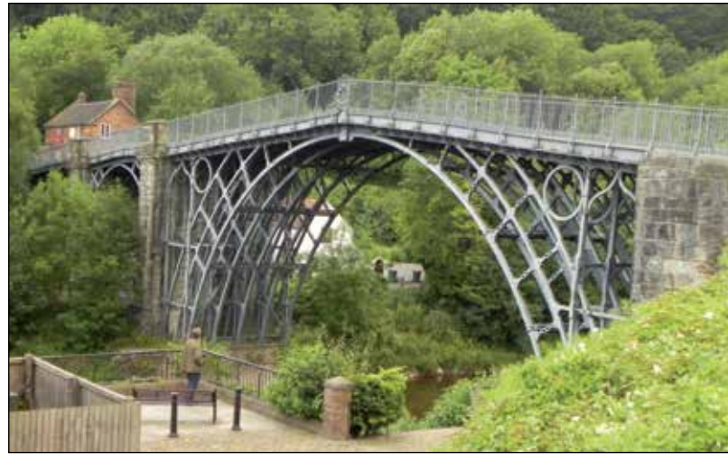
Figure 11.2. Ironbridge. The village Coalbrookdale in Shropshire in Great Britain, with its world heritage bridge built 1776-1779, is today a symbol and considered the cradle of industrialization in England and in the world. The preconditions were ideal for this early development – with iron ore mining in the area, a new method to produce coke from coal, and the river Severn flowing into to Bristol Channel. The surrounding landscape is a rich agricultural landscape providing the life support of the emerging industry population. Photo: Klara Livsey Berg
